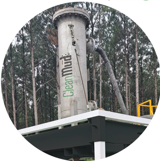
CleanMud Filtration System
